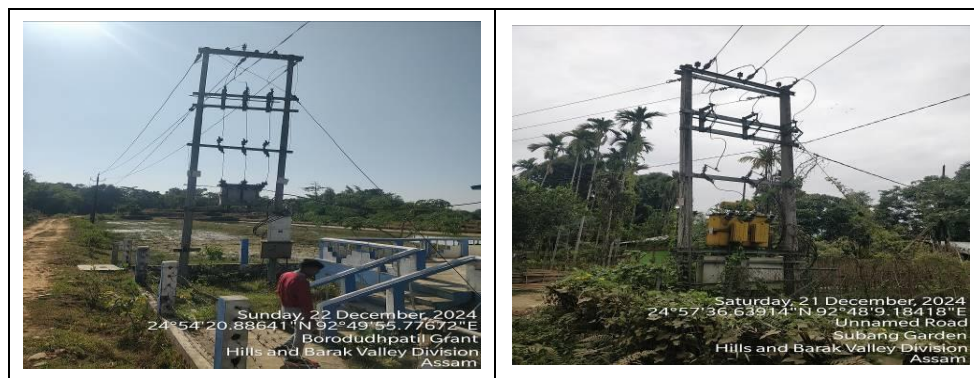
Figure 3-30: Electric Supply Facility in the Study Area
